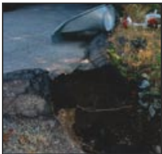
Before: Damage at end of road becoming serious.
